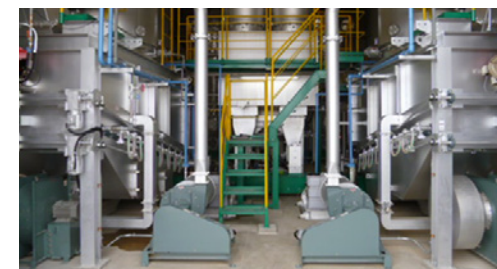
Biomass boiler at Odate Plant
